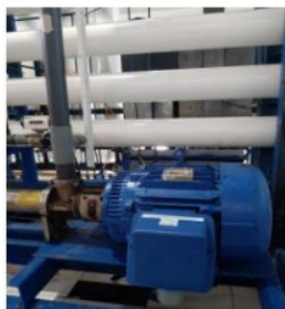
Gambar 10. High Pressure Pump (HPP).
